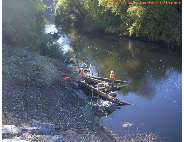
Above Right: Summer 2009, Construction is almost complete with the Boulder Wing Deflector in foreground, Live Willow Brush Mattress in the center and on the right, the Fish Habitat structure just below the Rock and Willow Lifts.
