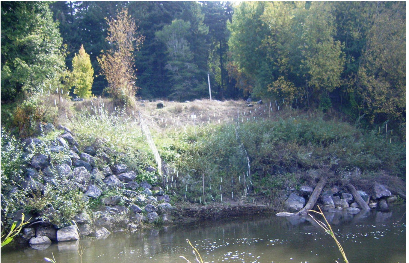
Above: October 2010, One year after restoration. Vegetated Boulder Deflector on left, Woven Willow Wall and Live Willow Brush Mattress in center and Log/Boulder Fish Habitat Complex on right anchored under Rock and Live Willow Lifts. White flags identify deer exclusion fencing
