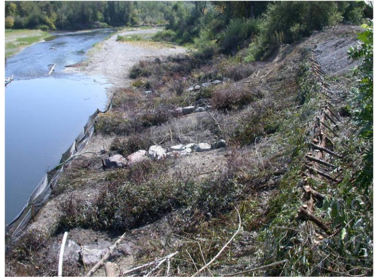
Above Right: Summer 2006, During Restoration: Live Willow Siltation Baffles and Live Willow Wall.
